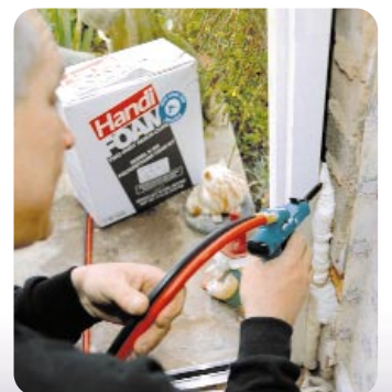
Handi Foam being used by Wyre Forest Housing Association for general doorway repair.
